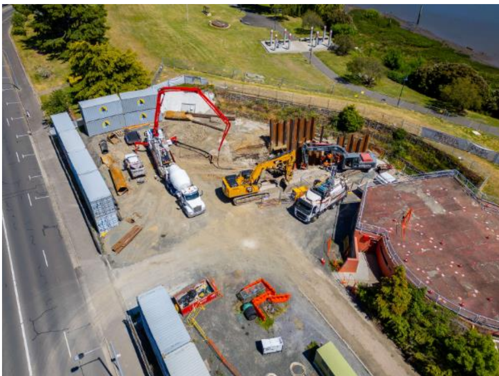
Recent works to connect the end of the pipeline drilled under the Tamar Estuary to the Margaret St pump station
