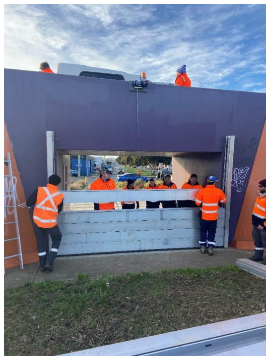
Closure exercise of Holbrook Street Gate/ Telstra gate (IG2), placing one of the logs in place
