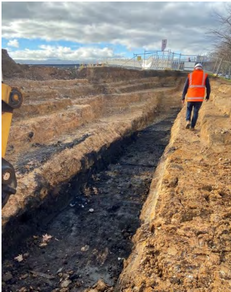
Figure 4 - The fully excavated levee section, showing steps along the sides and changes in soil/ clay composition
