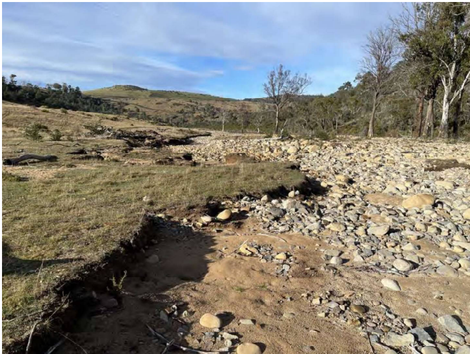
Figure A4-7: Evidence of previous water erosion from past flood events along the banks of the North Esk.
