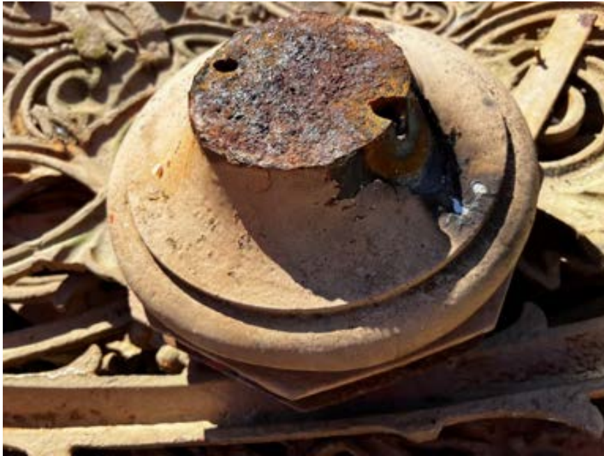
Figure 21 Showing the damage done to the crown trying to remove the Eagle Finial retaining bolts. These had corroded and swollen to such an extent, that they started to crack the casting.
