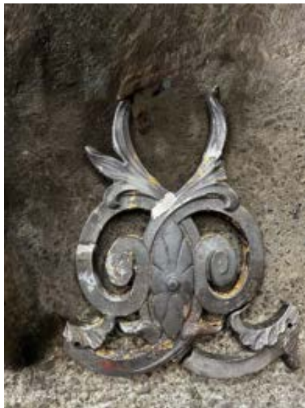
Figure 121 Photo showing broken section to be used as a pattern this will be cast in ductile cast iron
