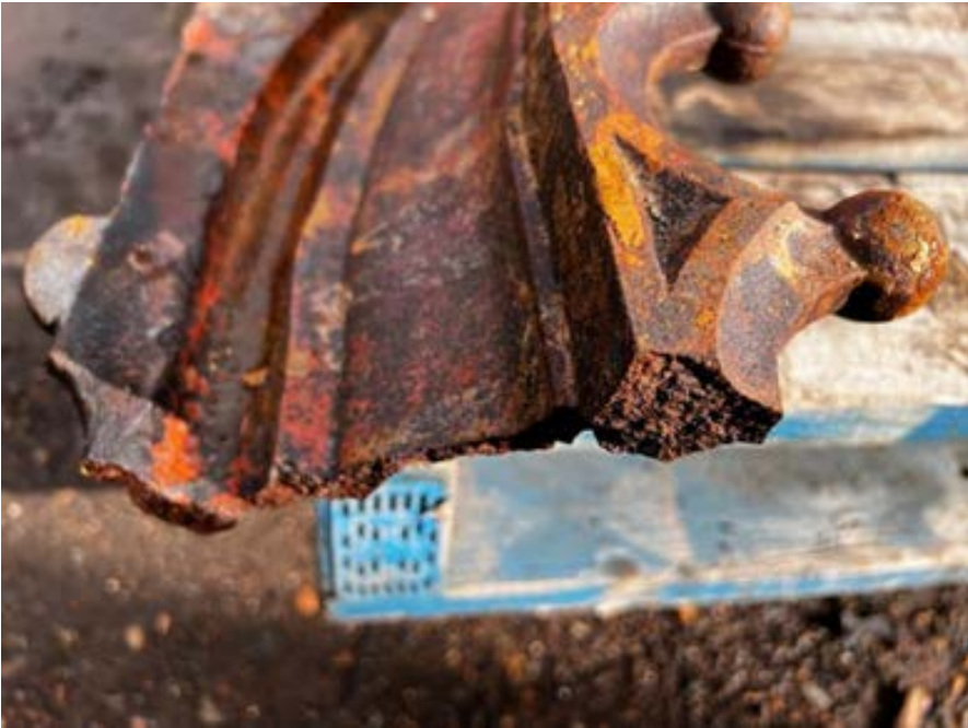
Figure 44 Shows number 1 of 4 broken sections on the Cusped Arch Front Face Panel where the plug attaches.
