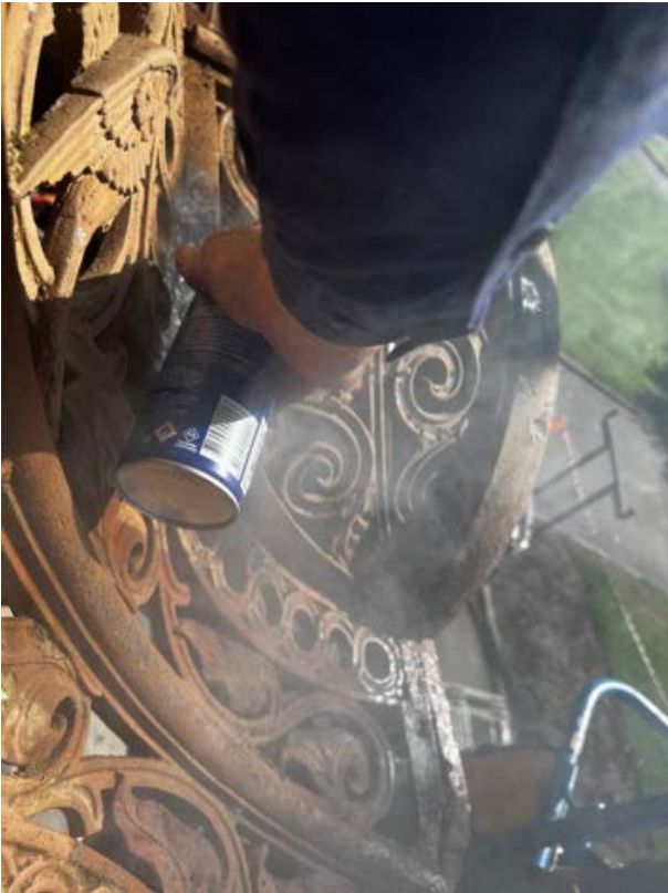
Figure 27 Photo showing us using heat and a combination of CRC and Yield to remove the screws
