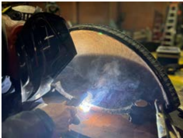
Figure 78 Photo showing welding the cracks in the bowl with Nickel Cast electrodes
