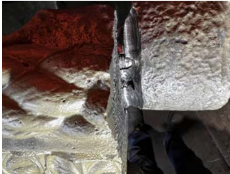
Figure 105 Photo showing crack being die ground out down to the two stainless steel bolts
