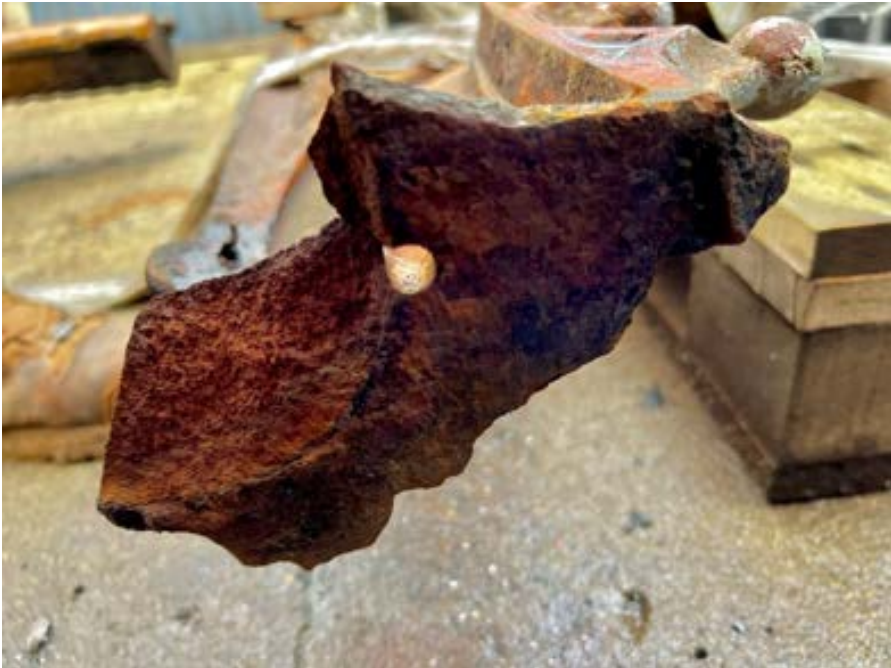
Figure 46 Shows number 3 of 4 broken sections on the Cusped Arch Front Face Panels where the plug attaches
