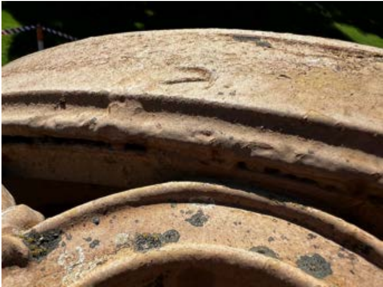
Figure 26 Photo showing the condition of the countersunk retaining screws trying to be removed
