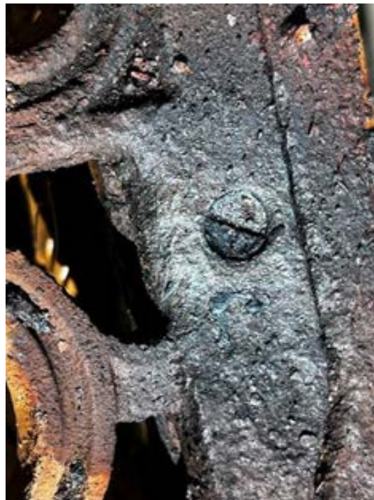
Figure 29 Typical screw condition found when removing the pendentive
