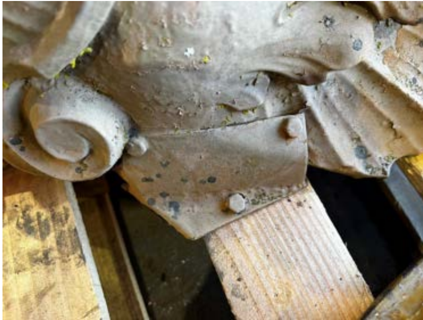
Figure 11 Showing broken Griffin Terminal this one wasn't even fixed to the canopy pendentive, it was just sitting in position and could have fallen off at any stage.
