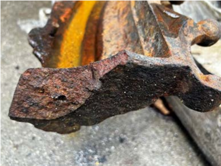
Figure 45 Show number 2 of 4 broken sections on the Cusped Arch Front Face Panels where the plug attaches
