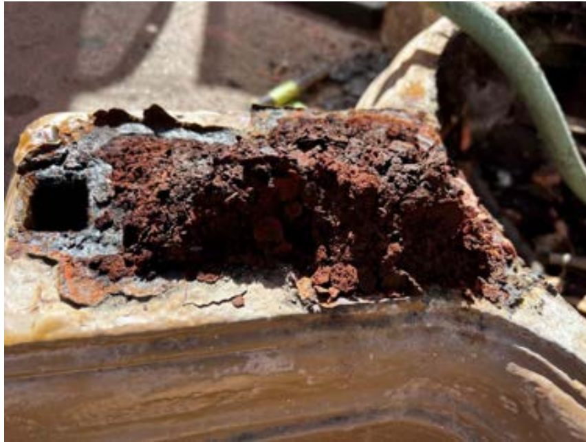
Figure 50 Photo showing the amount of rust that has come from the internal sections of the drinking fountain. We will sand blast and undercoat all the internal sections of the drinking fountain so this can't happen again
