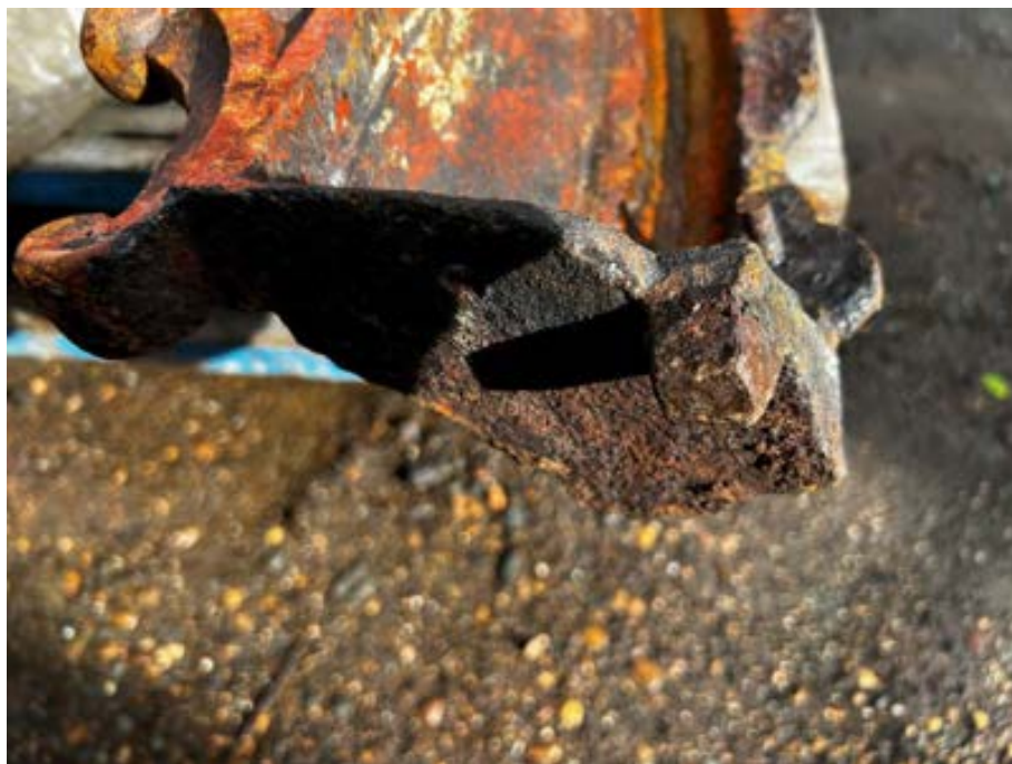
Figure 41 Photo showing locating peg on the other side of the cusped arched front face panels. The locating peg fits into the square hole cast into the top of the plug. Some of the square holes have corroded through allowing rainwater to fill the columns causing a considerable amount of corrosion internally.
