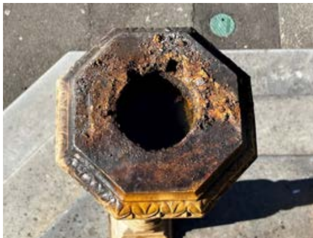
Figure 132 Photo showing the locating socket for the face panels, the holes corroded into the face panel plugs have allowed rainwater to fill the columns.
