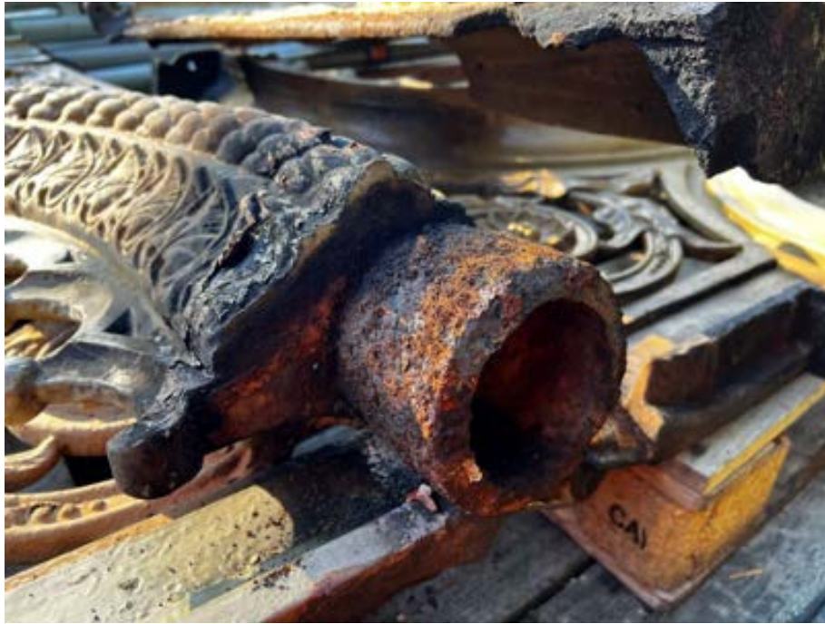
Figure 40 Photo showing badly corroded plug on the cusped arched front face panels, this fits into the socket cast into the top of the column
