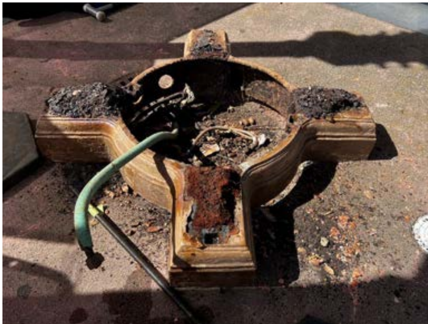
Figure 7 Shows the level of corrosion internally
