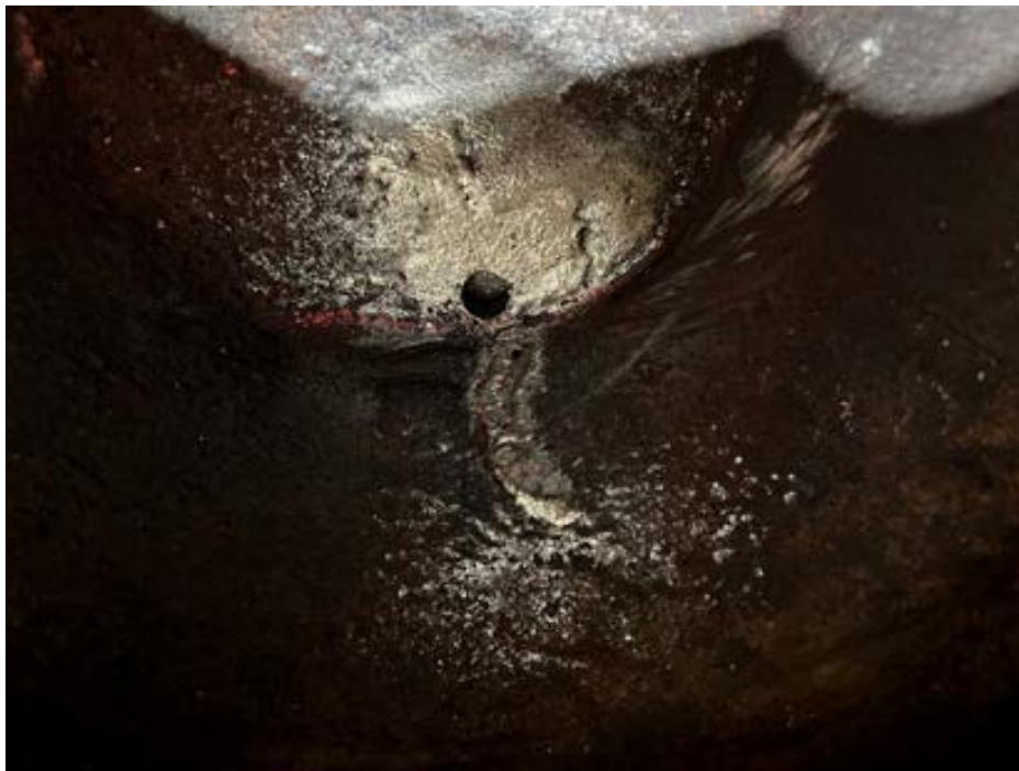
Figure 72 Photo showing cracks radiating out from the holes due to expansion of the bolts holding the eagle finial in place
