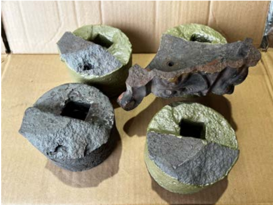
Figure 48 Shows the broken plugs from the cusped arch face panels. These are going to be the most challenging to repair due to the amount of weight they carry.
