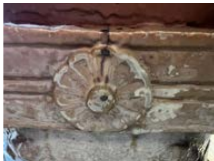
Figure 5 Shows all four straps were broken due to the level of base corrosion and possibly people standing on the drinking bowls over the years.
