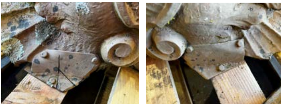
Figure 115a Photo showing the damaged Griffin with bolted on sections
