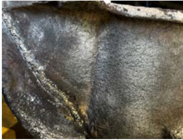
Figure 79 Photo showing repaired crack and peened weld on the bowl
