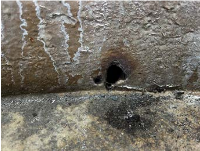
Figure 88 Photo showing existing badly corroded drain holes
