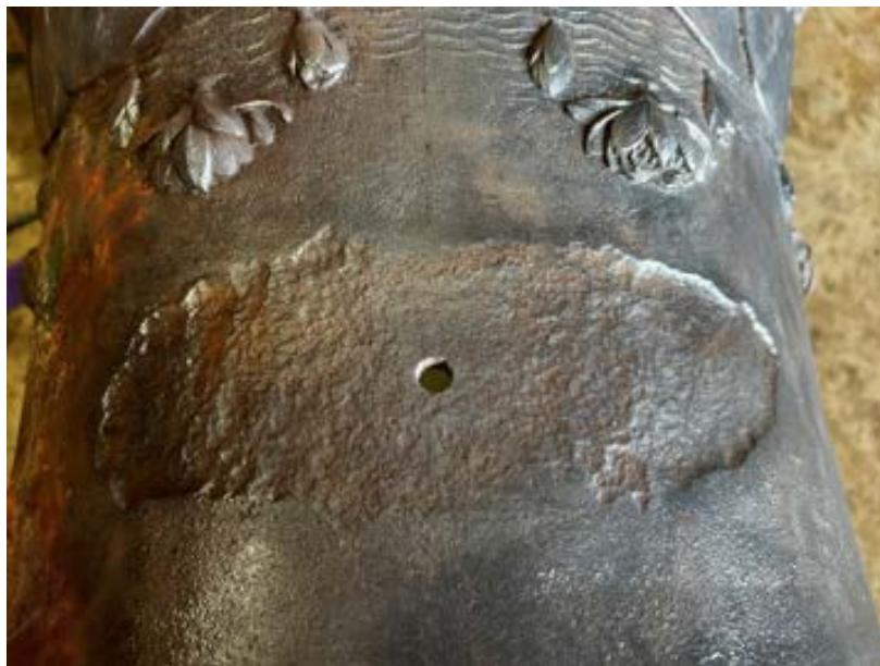
Figure 66 Photo showing the amount of surface corrosion behind the fountain main body support straps
