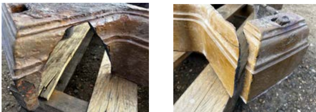
Figure 81a & b Photos showing the poor condition of the fountain base with broken, missing and corroded sections
