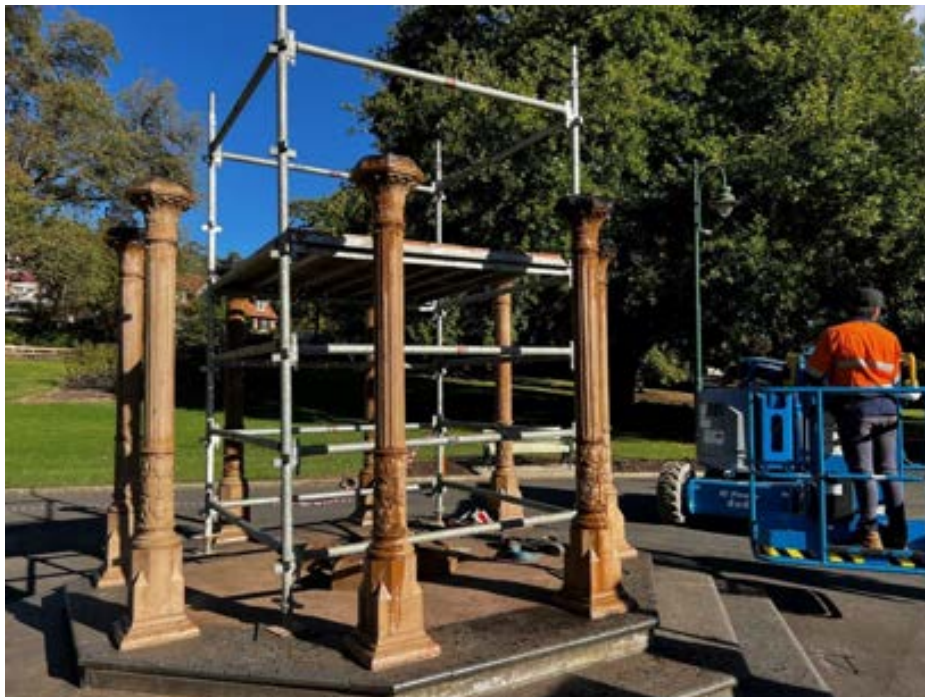
Figure 55 Photo showing the eight columns left on site ready to pump the rainwater out, strip and repaint
