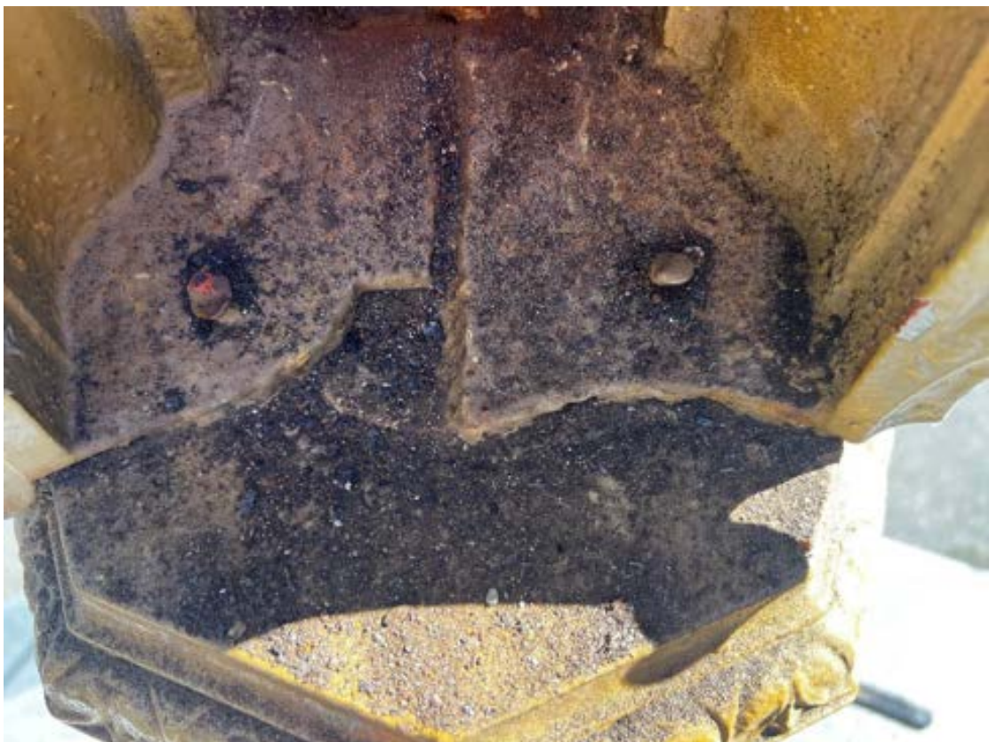
Figure 35 Shows two front face panels fitted on to the column, the panel on the right-hand side is the one with the round plug which fits into the socket cast into the top of the column. The panel on the left-hand side is fitted with a square tab that sits in the square hole cast in the top of the plug. The two locking pin heads can be seen prior to drilling out.
