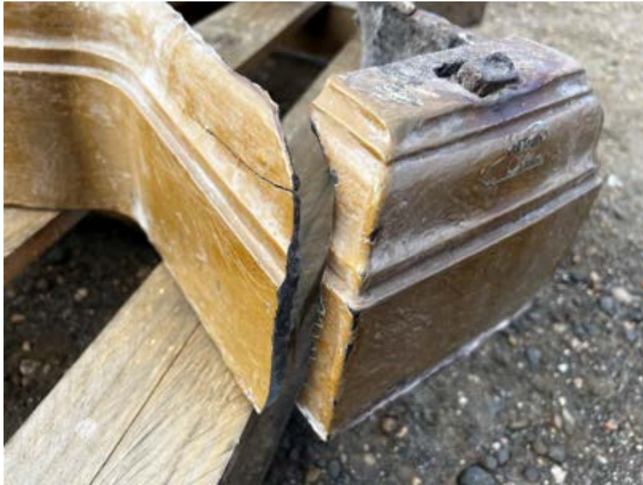
Figure 54 Photo showing historic broken section on the base plate, it also shows the locating tab corroded into the pocket and broken off the monopodia lion bowl support
