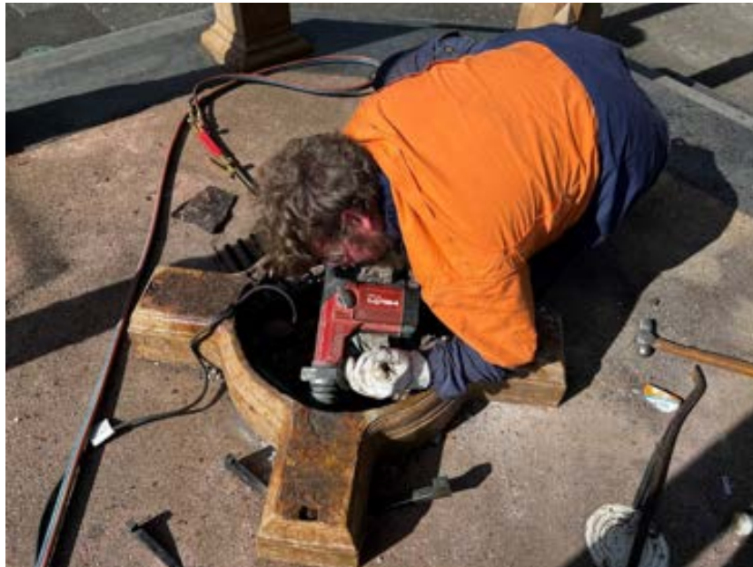
Figure 51 Photo showing Wes trying to remove the base plate by jack hammering the concrete and rubble with the Hilti. The base plate was cast into the concrete slab by 4 tabs at the outer ends of each arm on the base plate, these had to be cut off. The other option was to jack hammer the concrete, but this would have been a costly repair. It also had concrete, bricks, and rubble pushed into the outer extremities of the arm sections which had to be jack hammered out. We think this was done years ago to offer some support and help carry the weight due to the loss of material thickness through corrosion and breakages.
