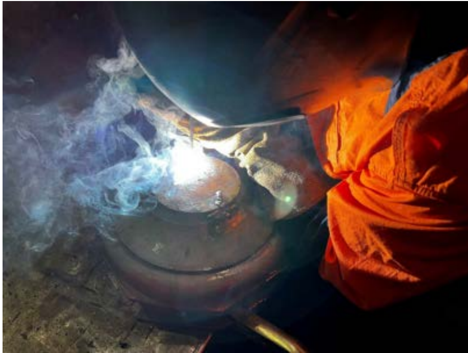
Figure 71 Photo showing the repaired hole and chasing cracks
