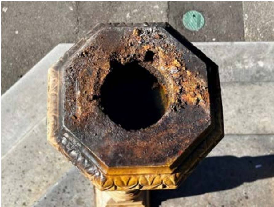
Figure 39 Shows the socket with the face panel removed the amount of rust we had to contend with made removal nearly impossible. Because some of the plug square locating holes on top of the plugs had rusted through some of the columns were full of rainwater.
