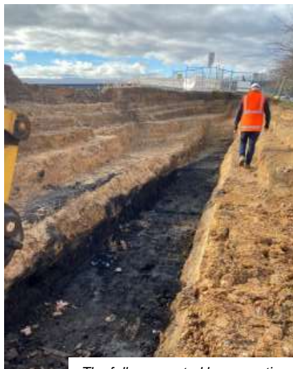
The fully excavated levee section, showing steps along the sides and changes in soil/ clay composition
