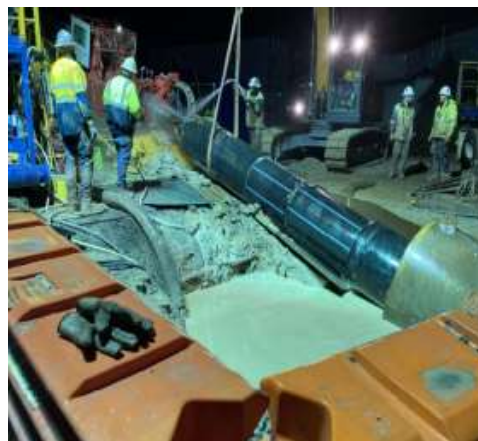
Final pull through of one kilometre section of pipeline to Margaret Street pump station. (Photo courtesy TasWater)
