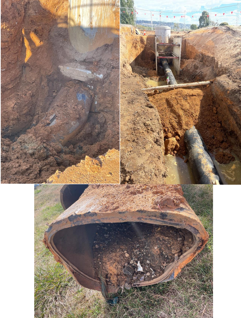
Top left - Damaged Pipe Top right - Replacement pipe Bottom - Damaged pipe after removal
