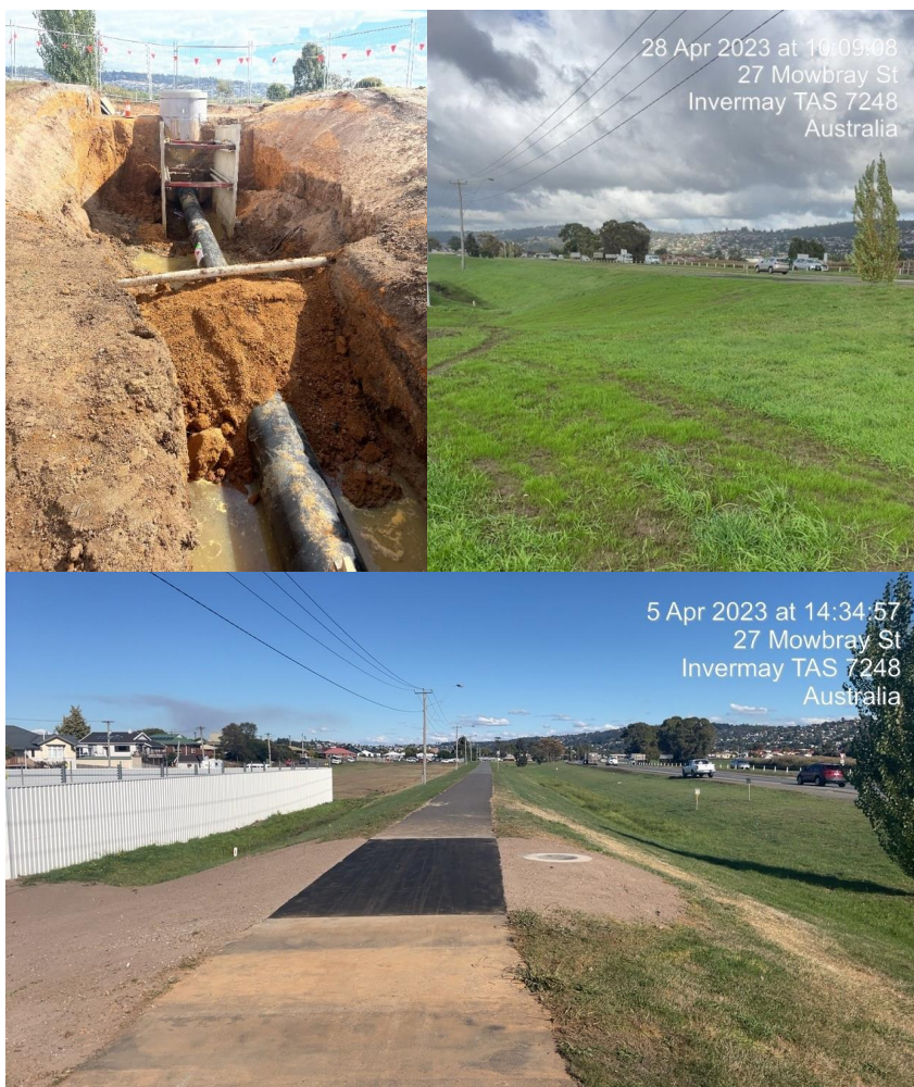
Top Left: New stormwater main after installation - 30 March Bottom: Reinstated levee after clay compaction and top soil - 5 April Top Right: Reinstated levee after work completion - 28 April
