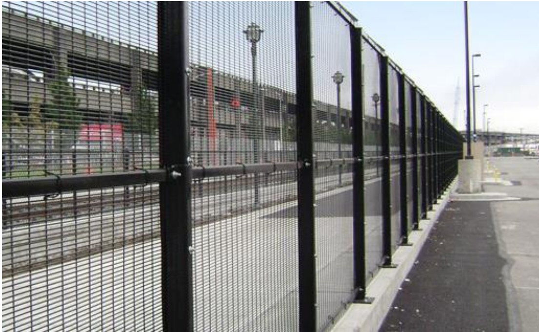
Figure 02: Image of fence installation utilising the same proprietary system. Note, fence proposed as part of this application will not require the intermediate structural member shown in this image.
