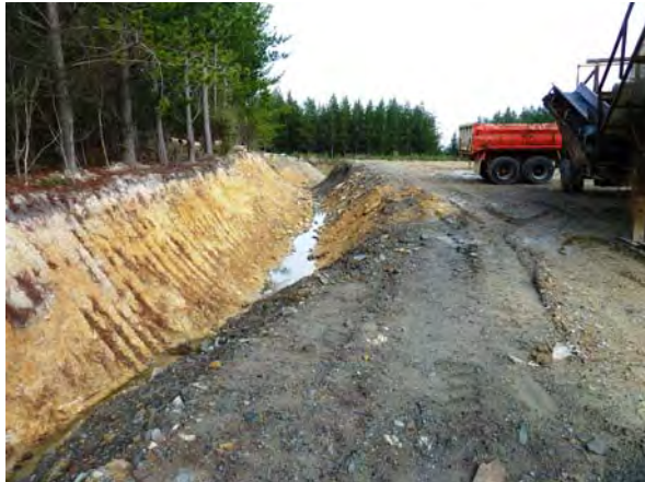
C. Road and drainage channel from existing pit to the existing sediment settling dam
