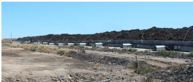
Figure 1: Aeration system at Jeffries Buckland Park, ADELAIDE (Jones 2015).
