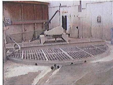
Concrete plant recycled water solids held in suspension by continual agitation (electric motor and paddle)
