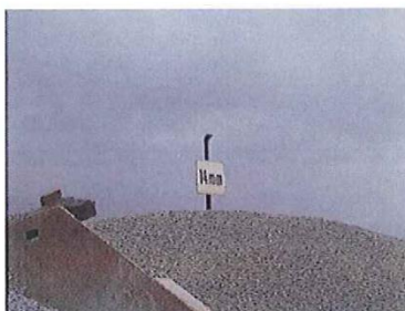
Concrete aggregate bins water spray system to reduce the effect of wind blown dust
